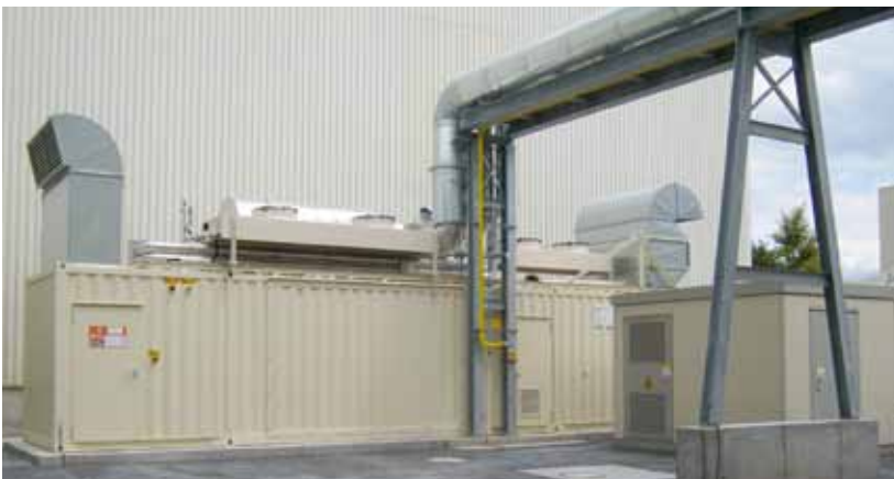
Decentralized power stations help to avoid energy loss.
